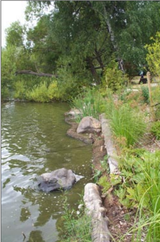
On the Green Lake shoreline, coconut fiber logs and native plantings were used to combat shoreline erosion and provide habitat. To suppress weeds and provide a healthy growing medium, high quality soil was brought in and compost was incorporated, then coconut fiber mats were placed on top and covered with a thick layer of wood chips.
