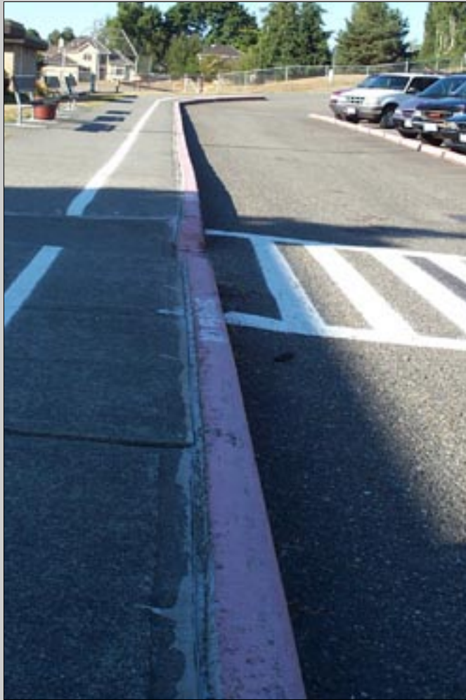
Weeds that grow in sidewalk cracks are often treated with herbicides because they are tough to tackle with manual controls. Here, cracks that were filled in have been maintenance-free for three years.
